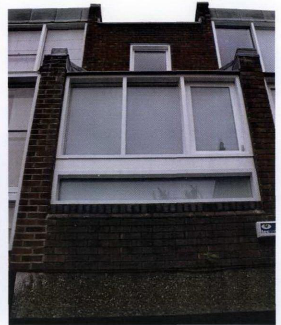
4 Lakis Close glazed balcony intended to be replicated.
