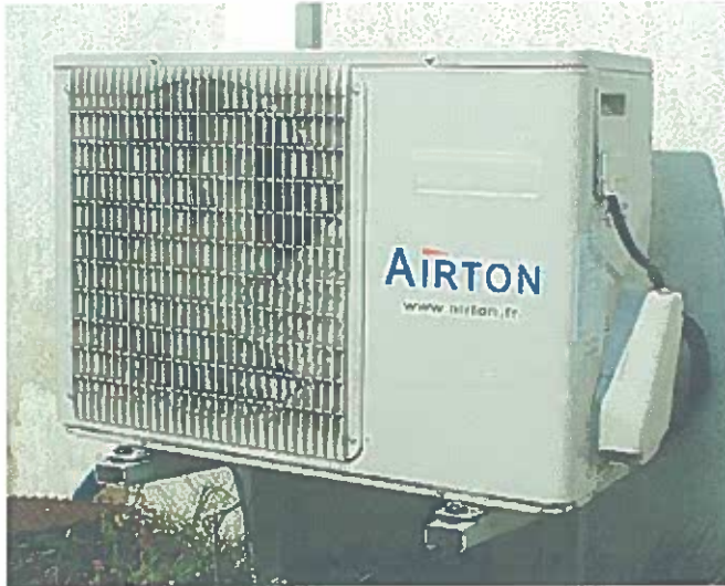
Fig 8: An Example of an external Air Source Heat Pump (Source: Internet)
