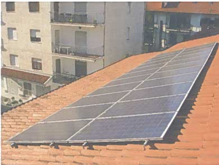
Figure 5: Roof Mounted Photovoltaic Panels (Creative Commons License)
