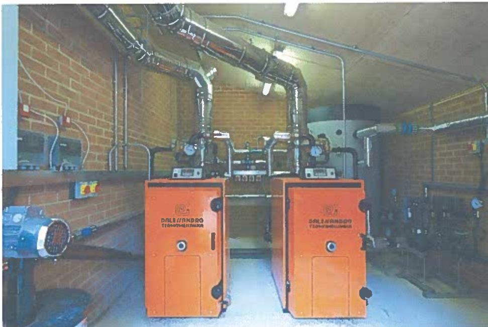
Figure 6: District Biomass System (© Ingleton Wood LLP)
