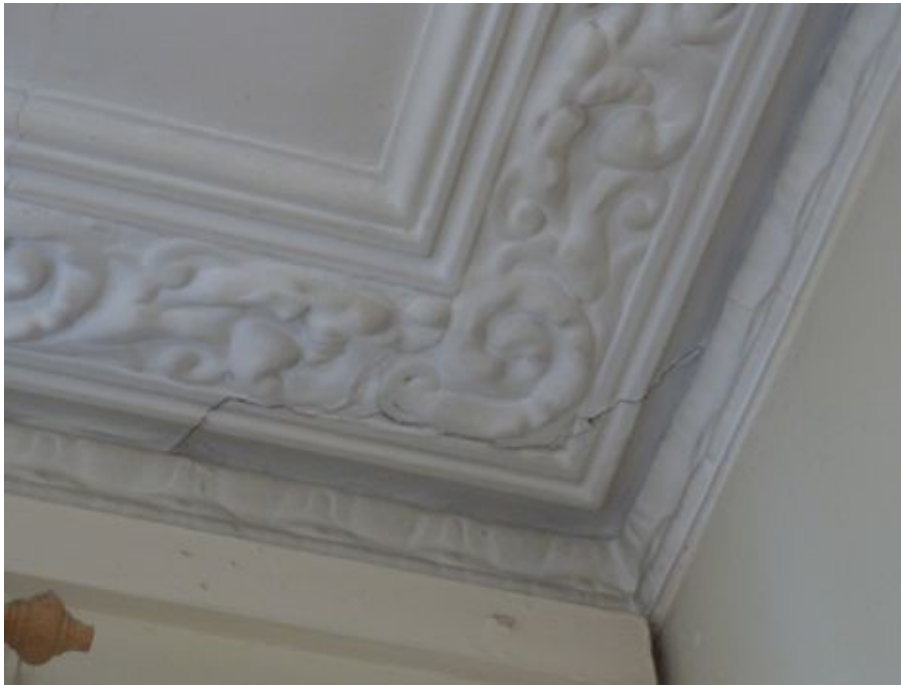
Fig.12 Existing overpainting and cracking to the principle room facing Princess Road
