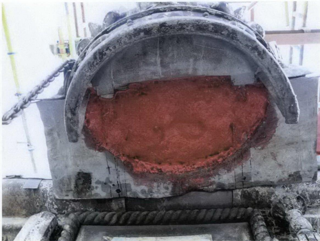
Figure 28. Crown filled with high density polyurethane foam
