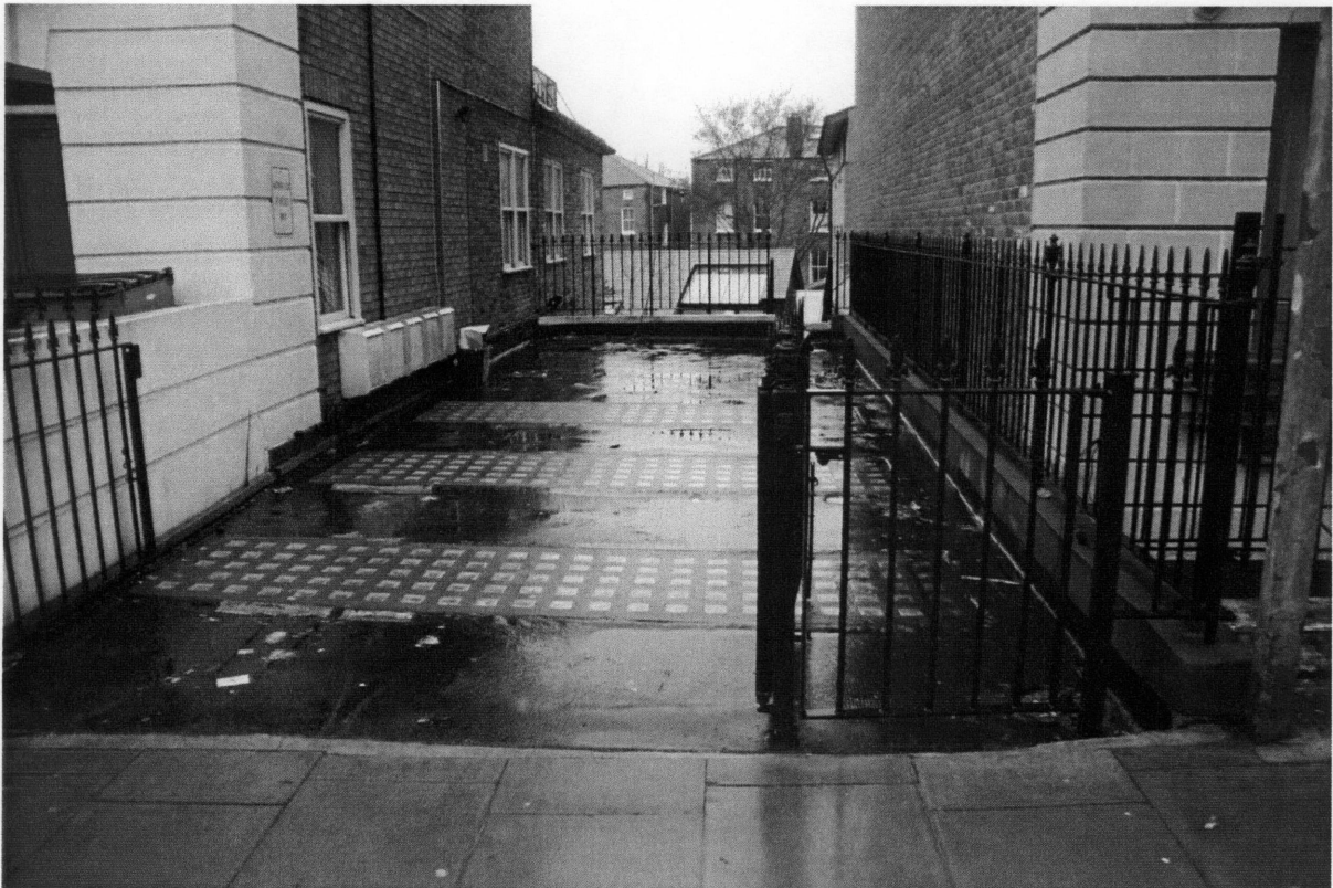
2) Existing parking area forming the roof of the existing underlying lower ground floor flat.
