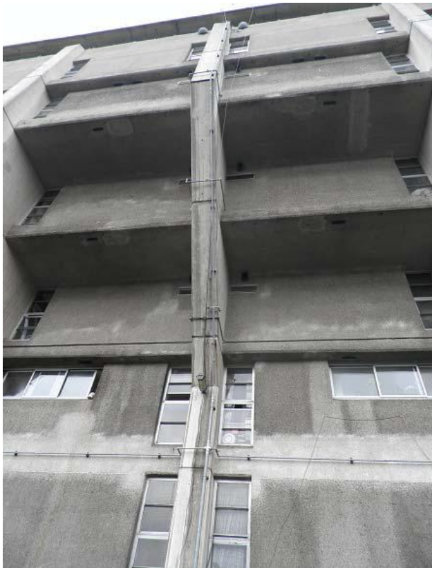
Figure Four: Block C – Building 54 External pipework installed in 2008 which is to be replaced
