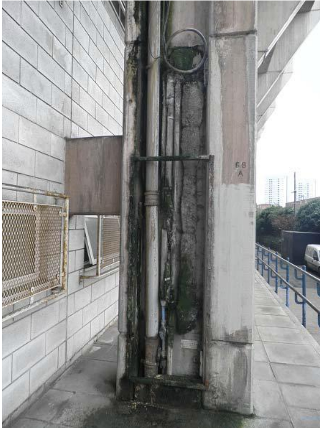
Figure Three: Existing gas riser within the service duct
