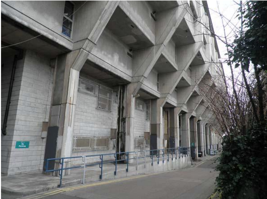
Figure Two: Block E (shop, council office and access road located under this block) showing the service ducts within the columns
