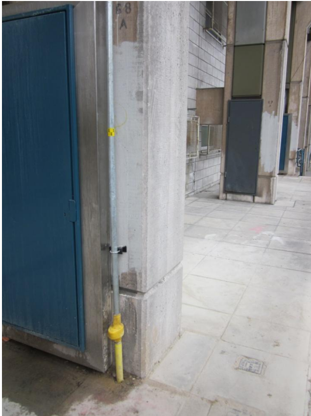
Figure Six: new gas supply and valve, showing standard fixing
