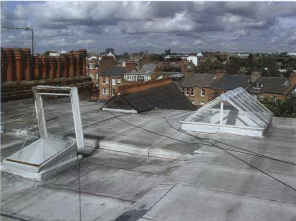
11 Existing roof showing existing access hatch and unprotected edges
