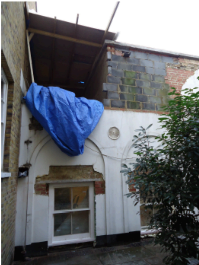
Photos from Private Courtyard to 12 Theobald's Road Image shows size of new terrace; height of existing parapet wall across section of new terrace
