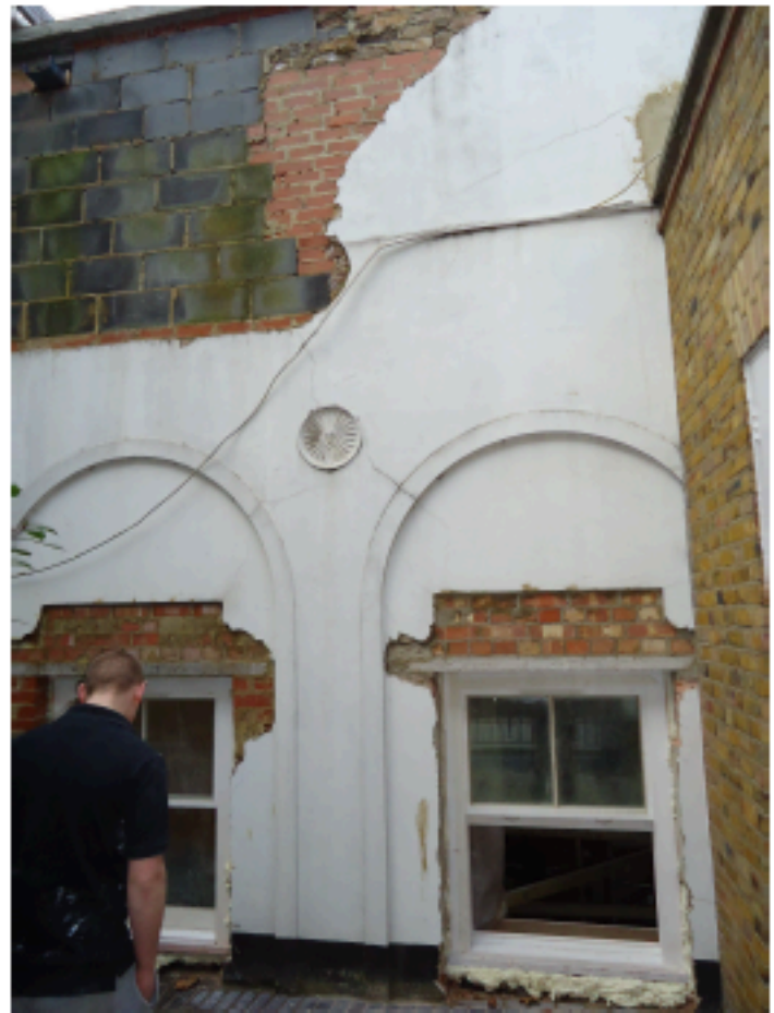
Photos from Private Courtyard to 12 Theobald's Road Image shows new windows fitted within existing openings
