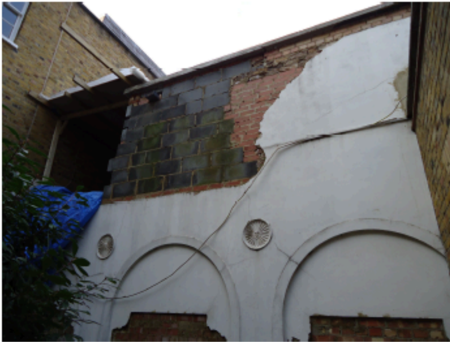
Photo from Private Courtyard to 12 Theobald's Road Image shows the existing, unforeseen render finish and decorative details
