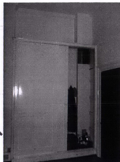
WITHIN EXISTING RISER
