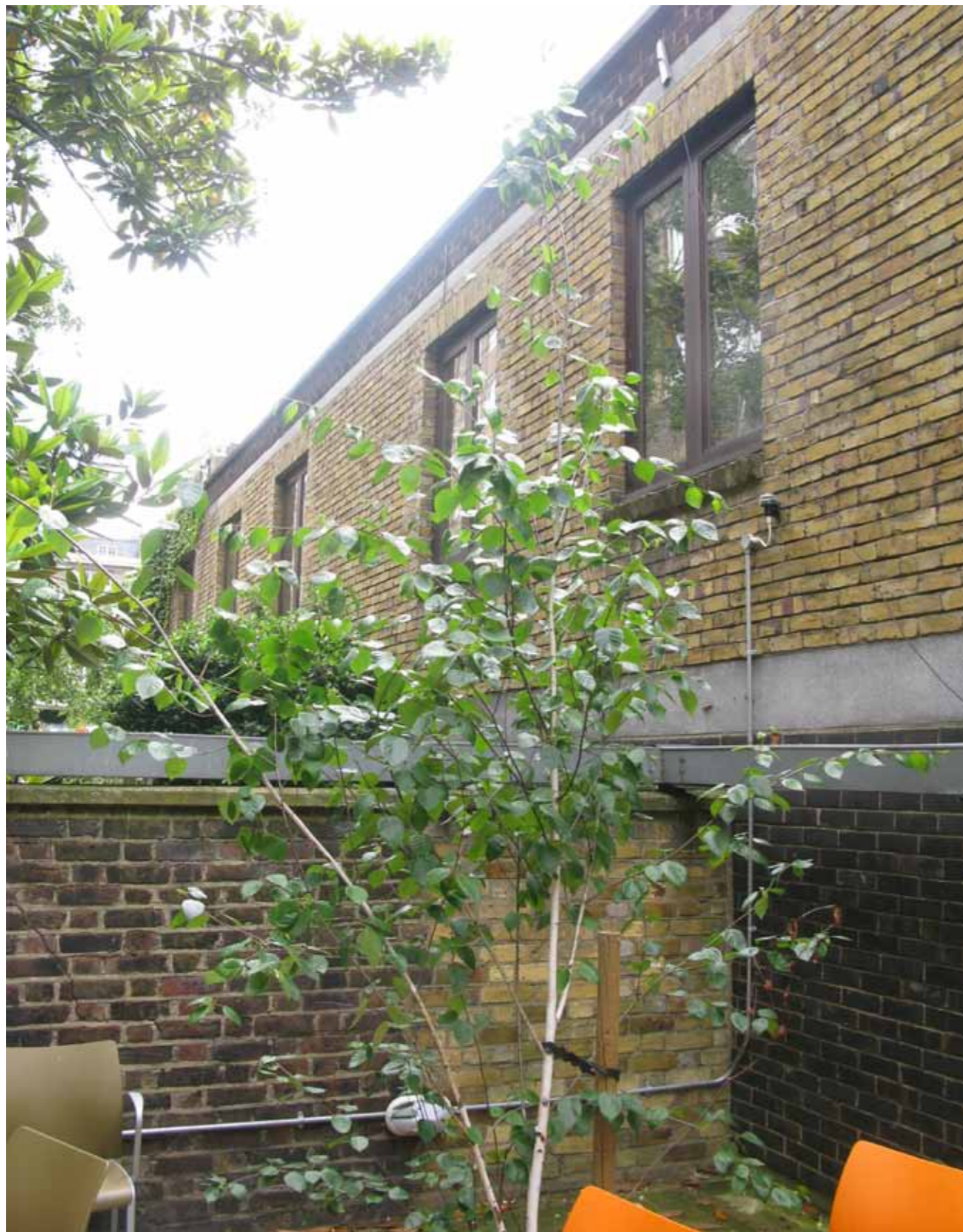
Rear elevation of mid 20th Century extension showing existing windows in the foreground (Photo taken from rear garden of 35 Tavistock Square)
