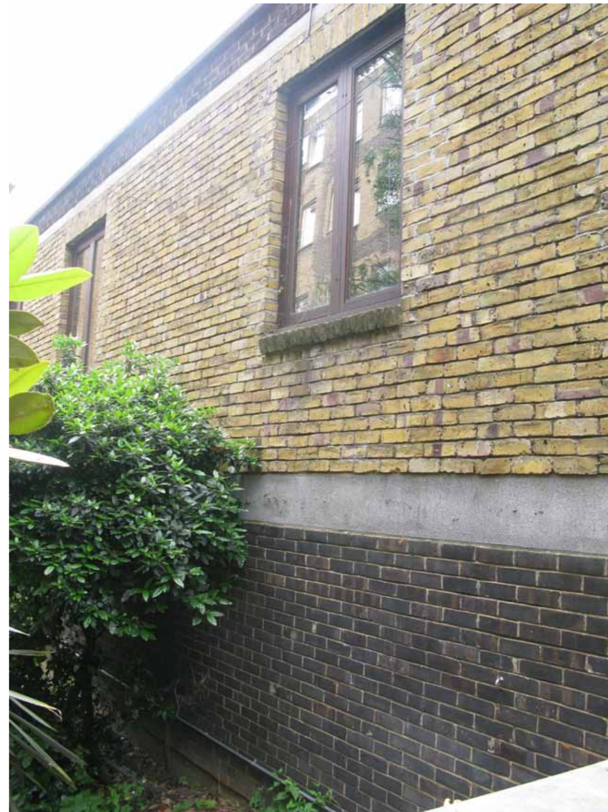
Rear elevation of mid 20th Century extension showing existing windows in the foreground (Photo taken from rear garden of 35 Tavistock Square)
