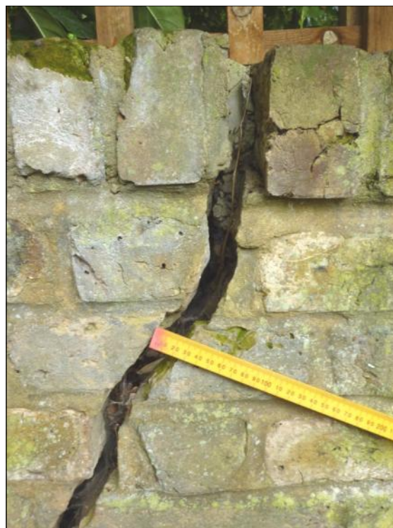
6. Photo of the crack in the wall near T3
