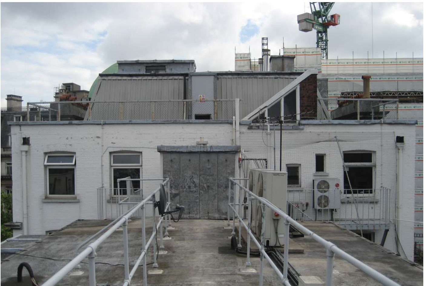
Photo showing the existing 5th floor roof area including condensers and water tank
