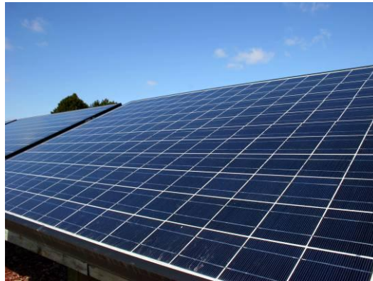
Figure 7.5 Photovoltaic (PV) Panels
