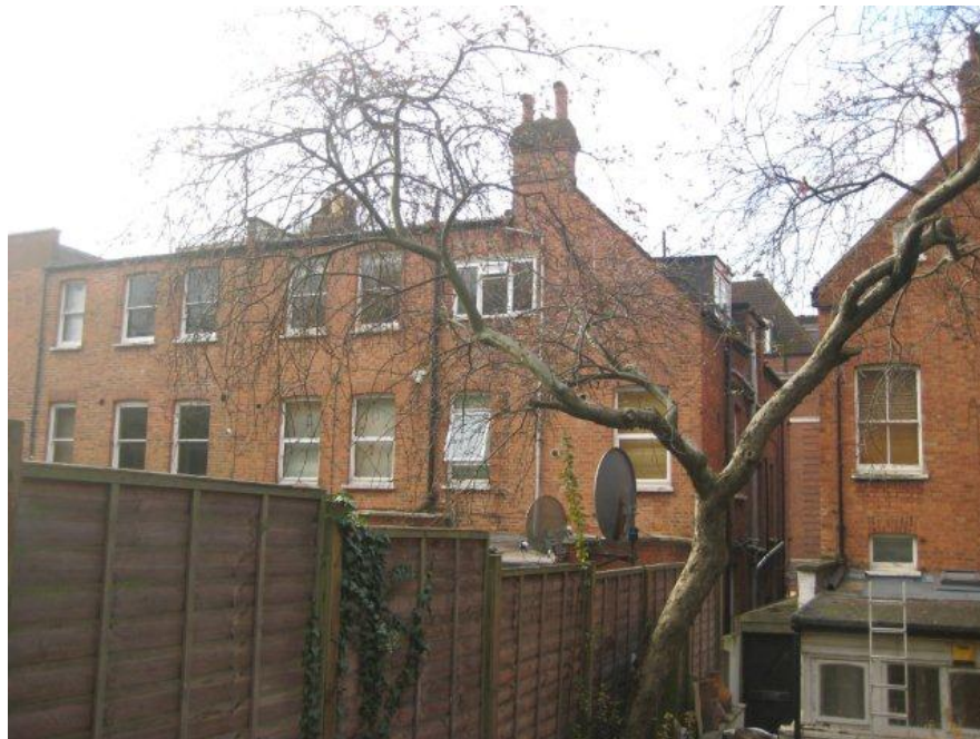
Rear of 224 Finchley Road showing existing mixture of uPVC and timber windows.
