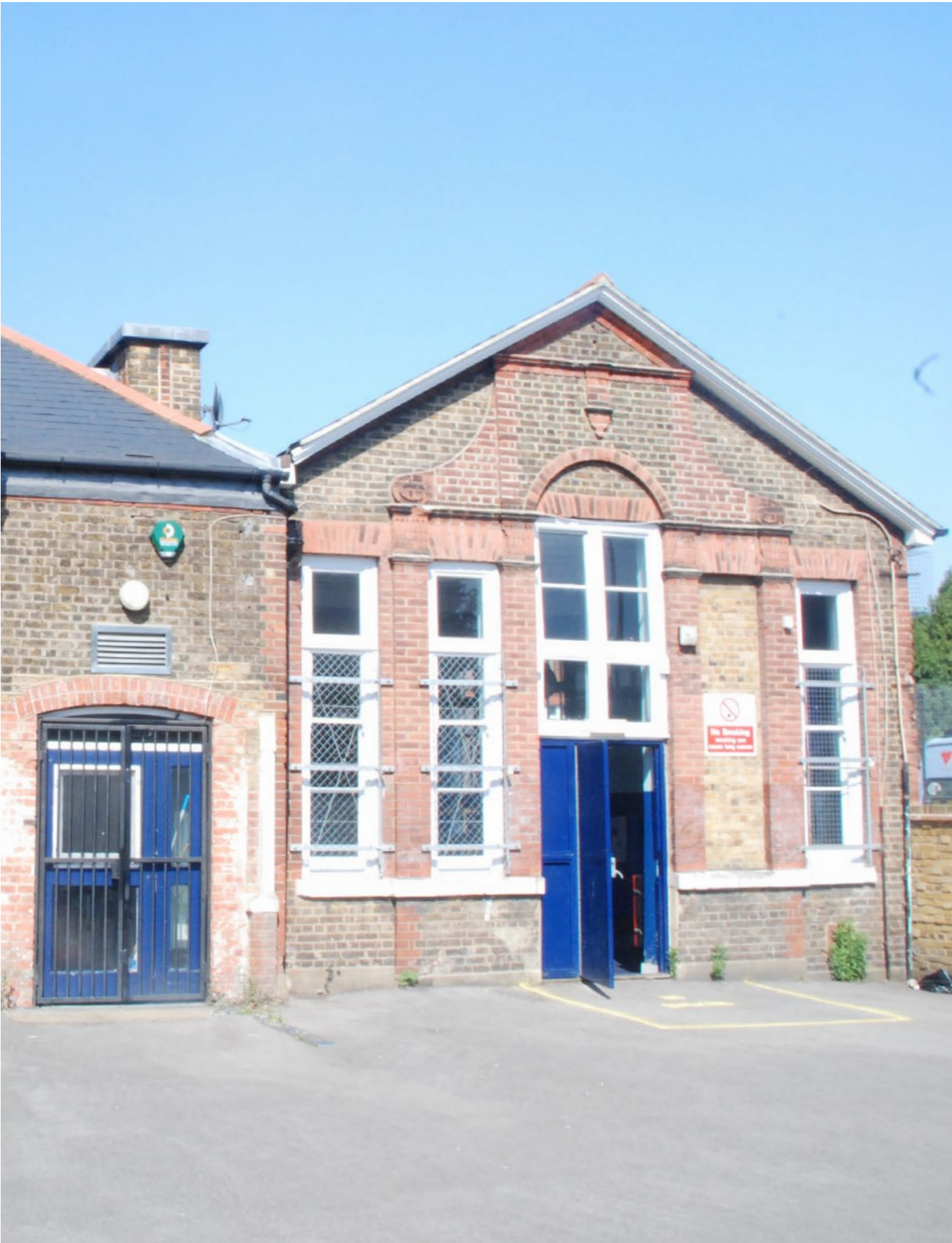
Existing sash windows are now inoperable. Large areas of South facing glazing causes significant overheating
