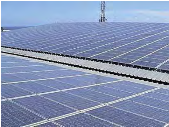
Roof mounted PV Panels
