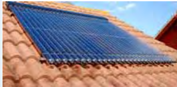
Evacuated tube collectors
