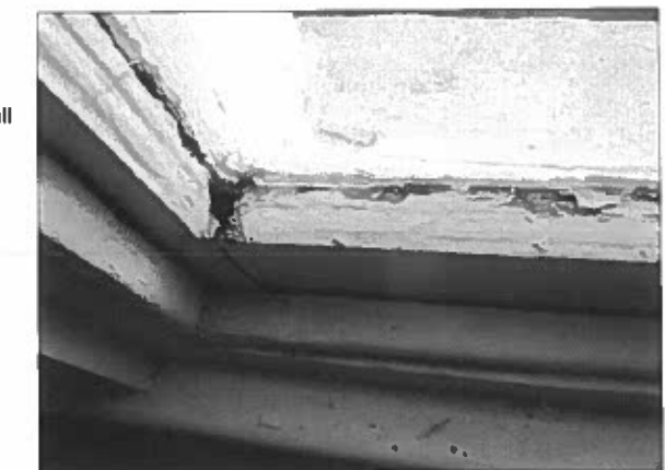
Investigation Work: Photograph showing rotten sash window WS02 needs replacing in like-for-like manner.
