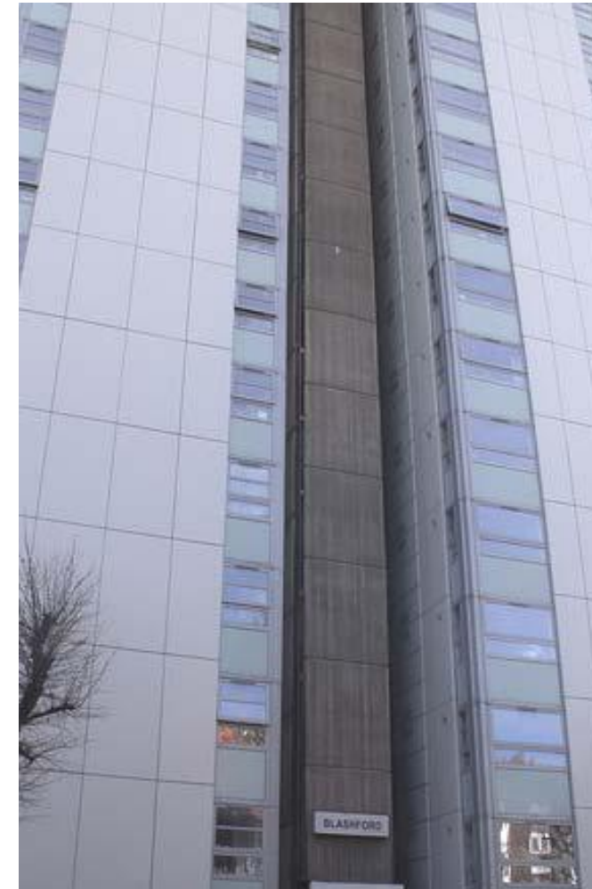
Blashford House after recladding. Part of the original ribbed concrete has been left visible.
