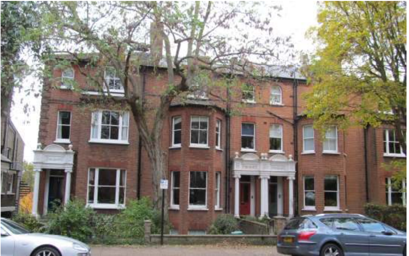
Photo 3 Front elevation of houses on Dartmouth Park Avenue Note 1 No signs of movement.
