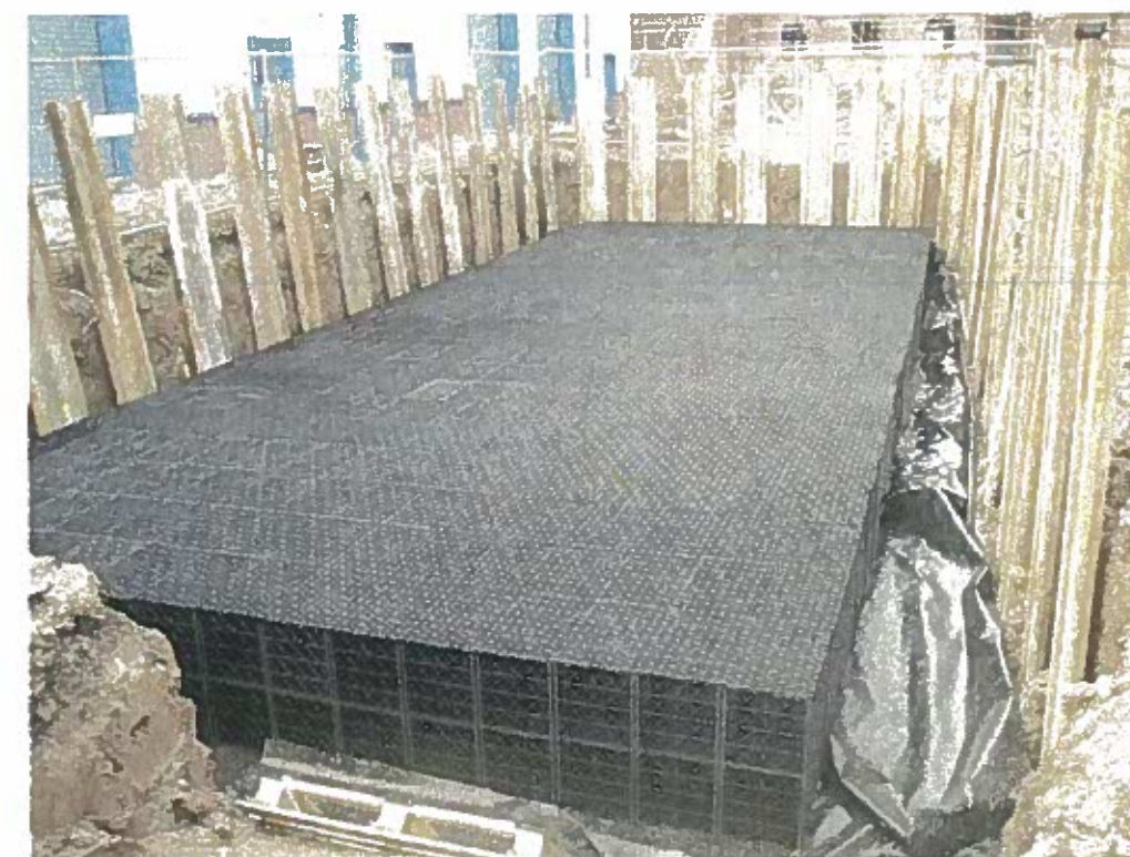
Example Attenuation Tank
