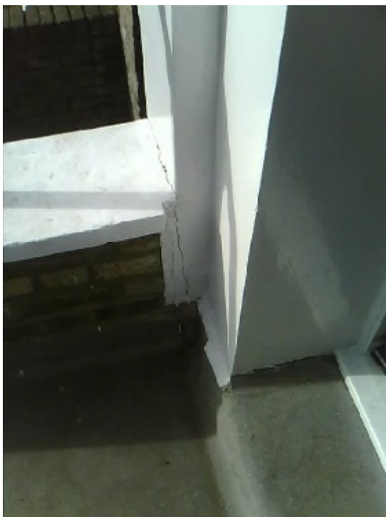
FIGURE 03 - Separation at the junction of the entrance steps and the main dwelling - High Level
