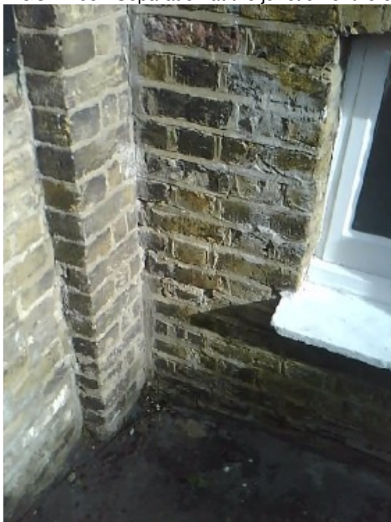
FIGURE 04 - Separation at the junction of the entrance steps and the main dwelling - Low Level
