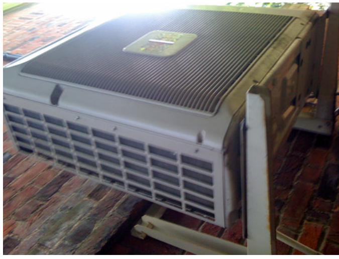
02 Existing Photographs of current external air conditioning unit located on Side Elevation (North) in side passage
