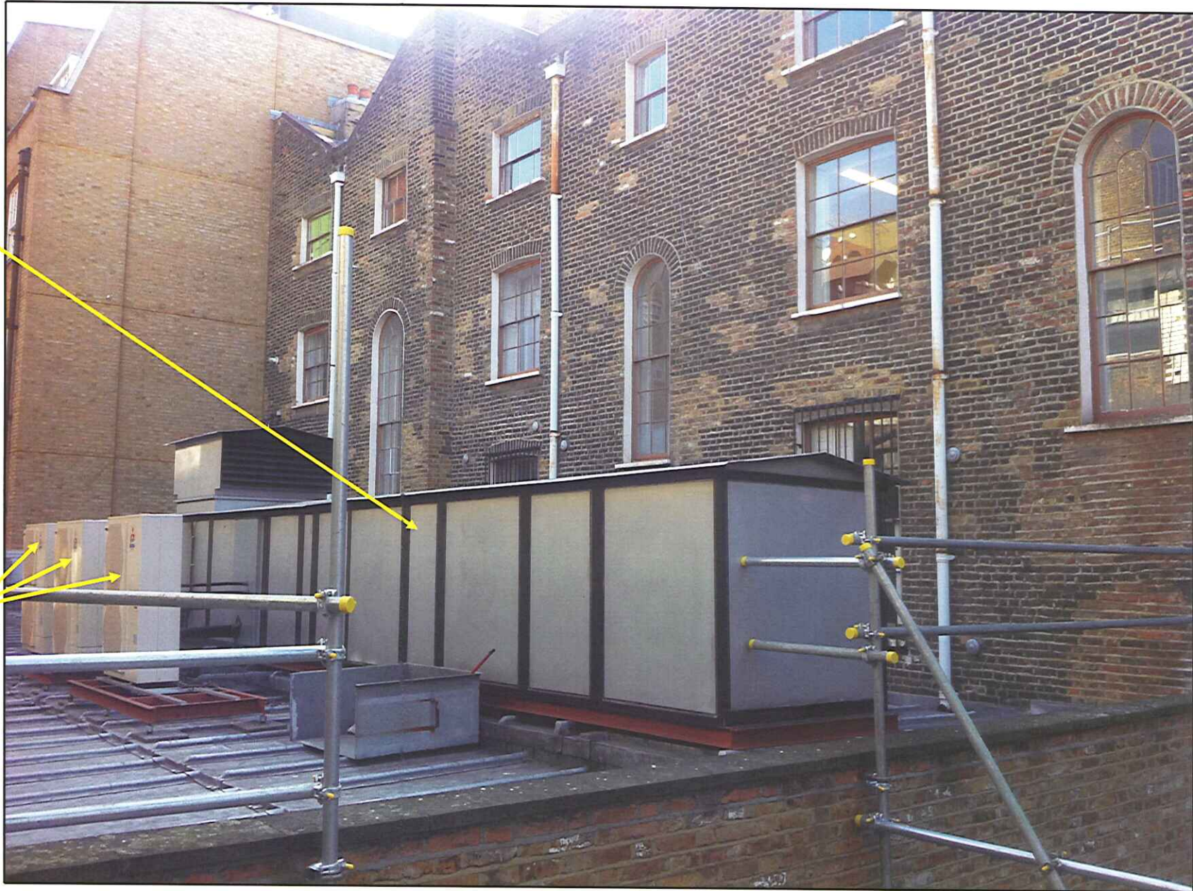
PHOTO C: Rear façade of Venezuela Consulate building with Air Handling unit and Condenser on first floor roof.
