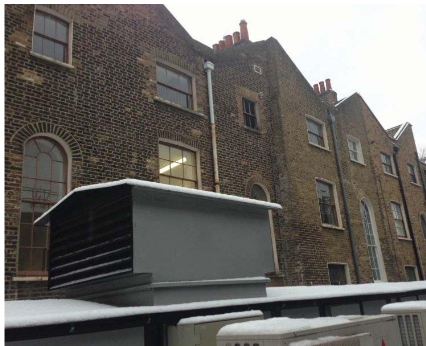
View to rear looking West showing plant on the roof of the Bolivar Hall
