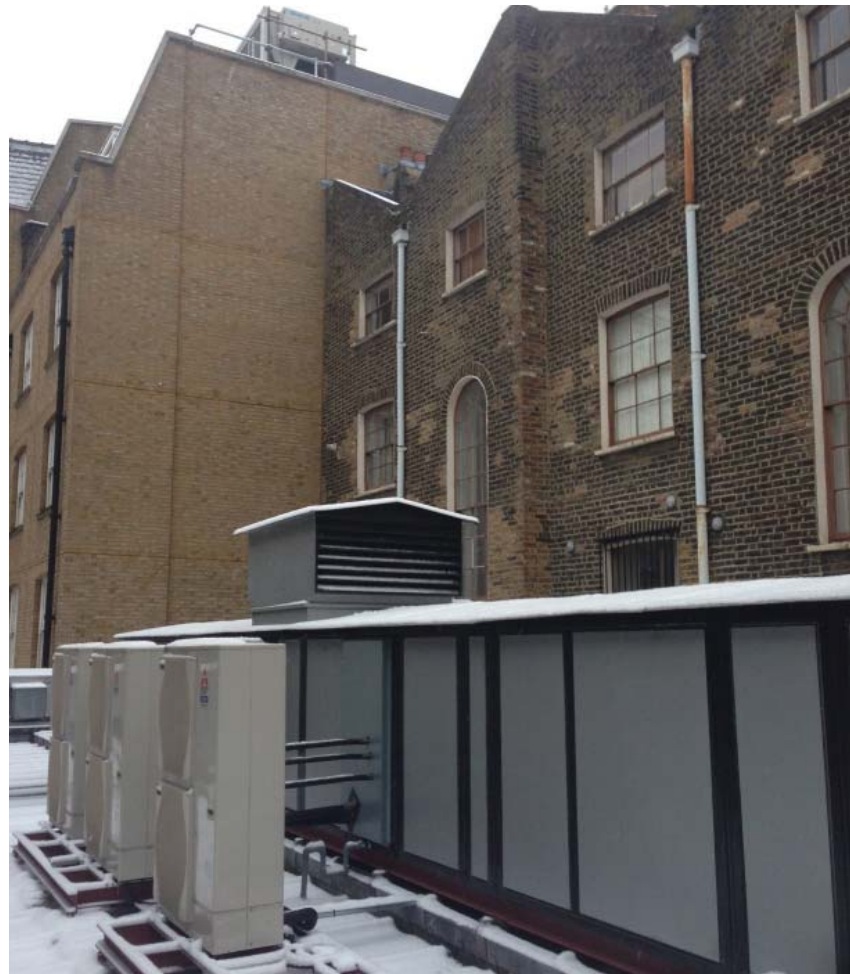
View to rear looking East showing existing large metal duct and separate plant units on the roof of the Bolivar Hall
