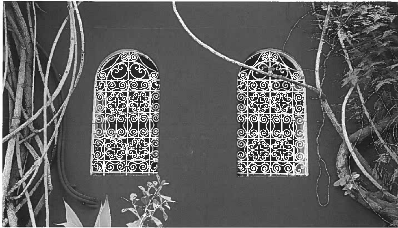
01 The Moroccan window uses a fine mesh to provide views out but not in
