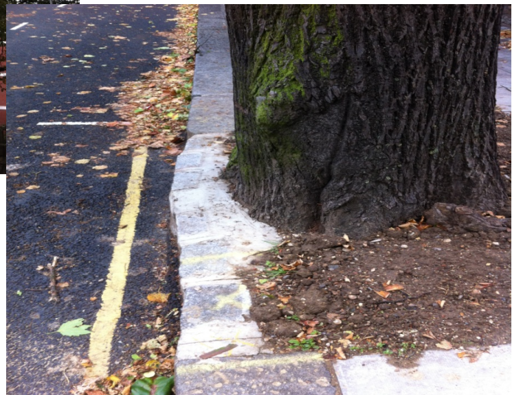
Tree2 – Root damage and disturbance following highway repairs
