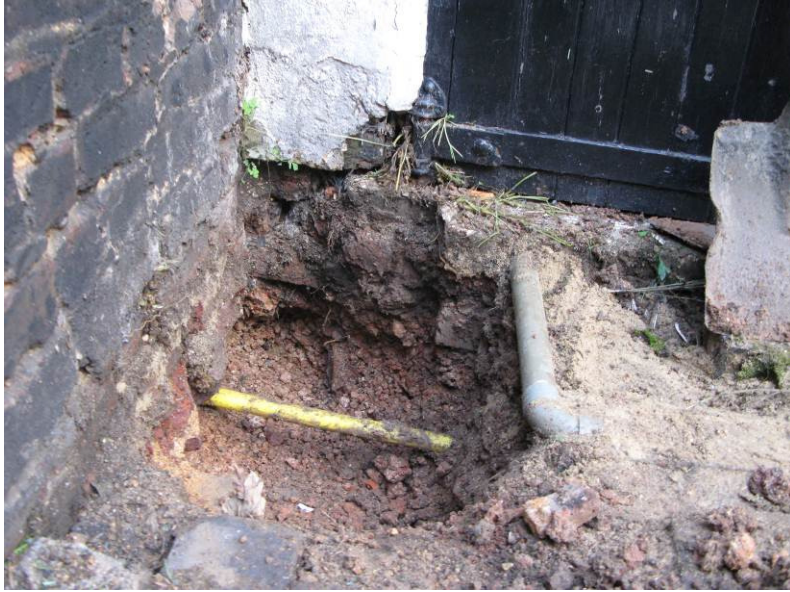
PHOTOGRAPH 5 Displaced dilapidated brickwork
