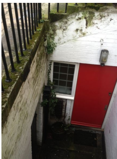
Vault entrance to LGF, replacement of door and window in line with neighbouring alterations. (REG/17-020)
