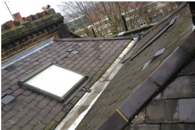
Roof view of existing roof light. Proposal to extend and to create a similar roof light adjacent to improve access to natural light. (REG/17-016)
