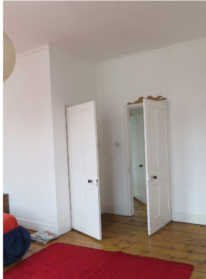
Existing view of Master Bedroom. Proposal to reconfigure and create direct opening to landing. (REG/17-014)
