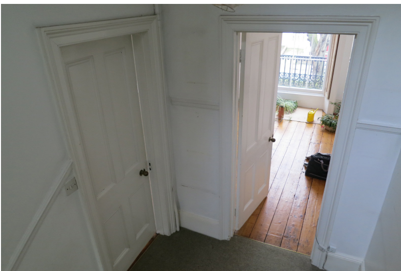
First floor landing. Proposal to close opening on the left hand side. (REG/17-013)
