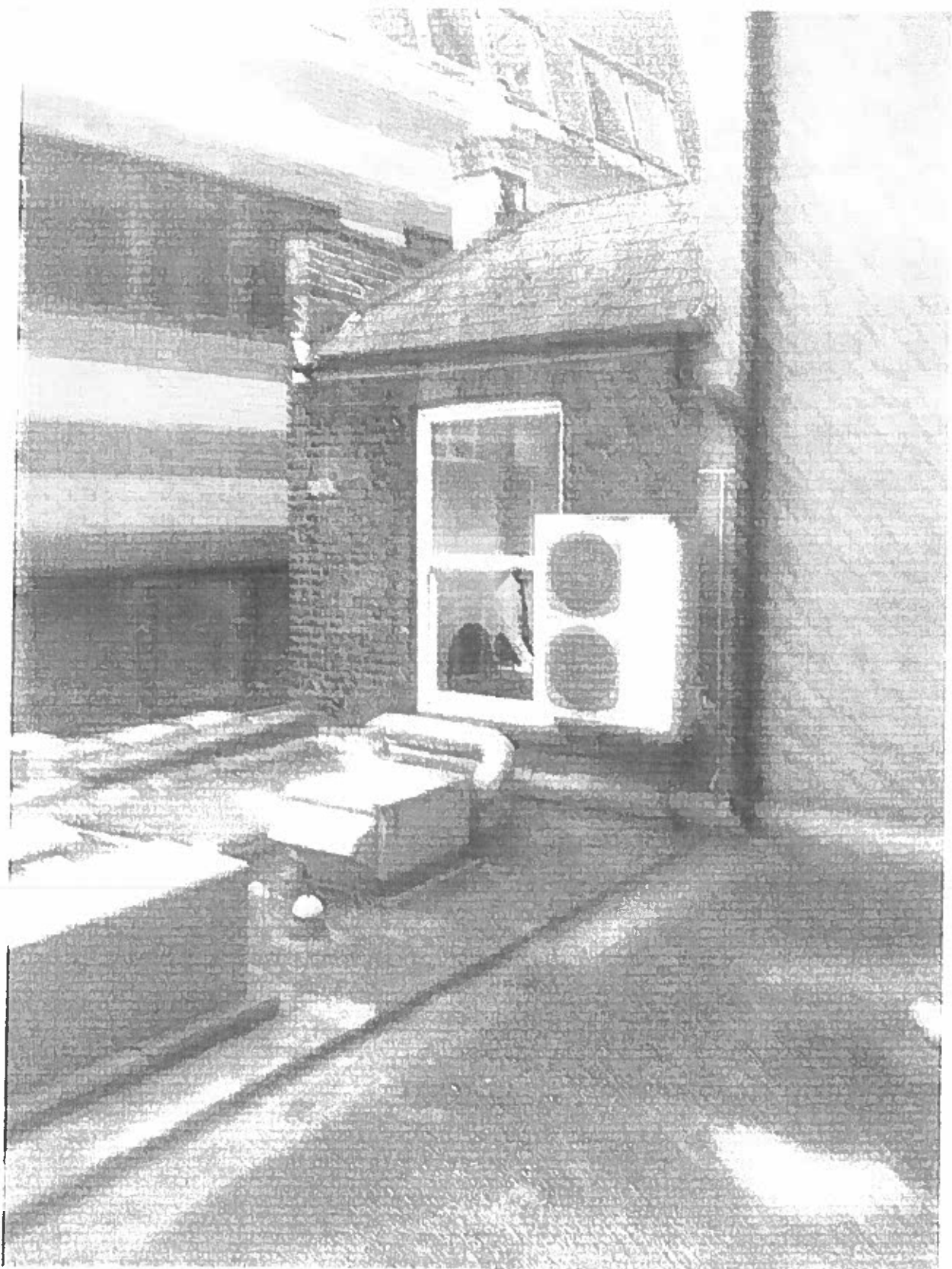
Photo E – Single Condensing Unit Owned by Tanfield Chambers Overlooking First Floor Roof (Switched Off During Testing.)
