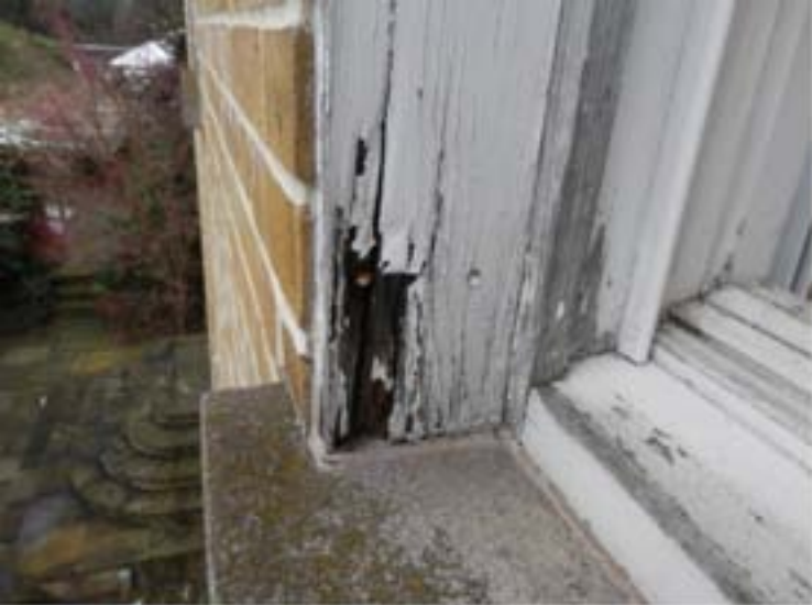
PHOTOGRAPH 25: ROT TO THE WINDOWS
