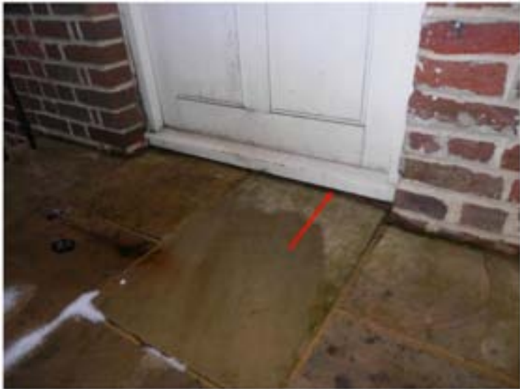
PHOTOGRAPH 21: NO WATERPROOF JOINT BETWEEN THE STEP AND THE WALL.
