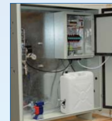
INTERIOR OF AUTOWASH CABINET
