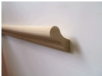
non-original mopstick handrail to be replaced with pigs ear handrail
