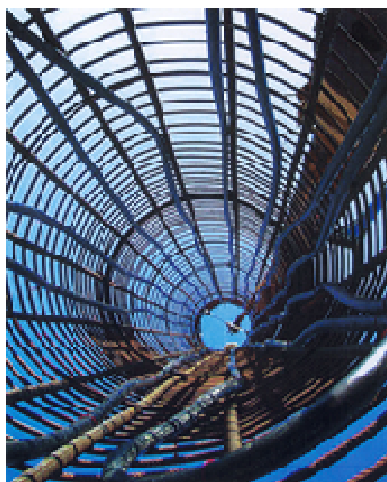
View down a ground source energy pile
