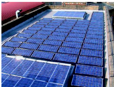
PV panels angled at 10° on flat roofs
