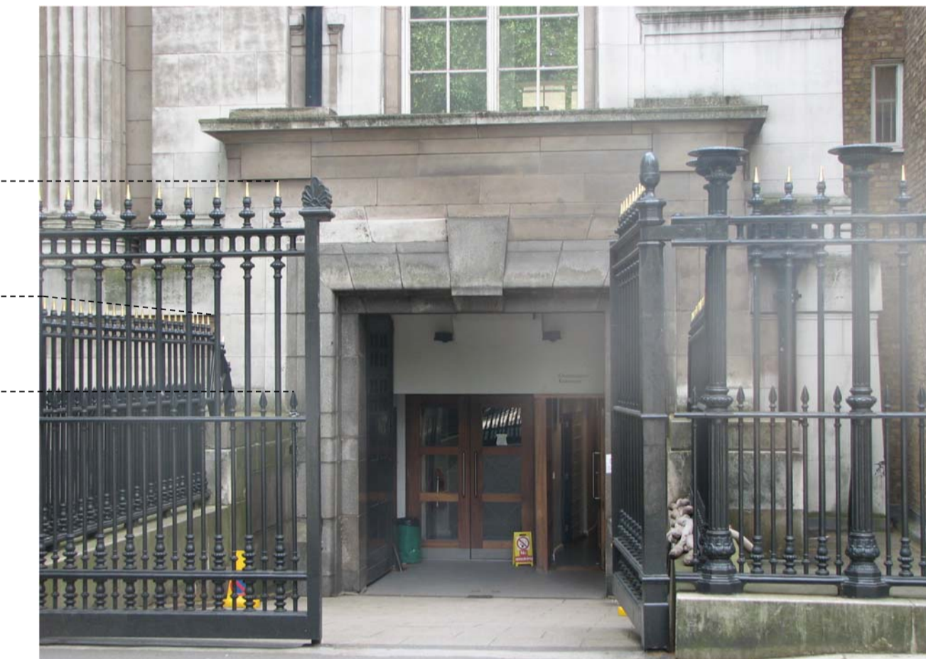
06 MONTAGUE PLACE RAILINGS A. Top of Montague Place railings B. Top of railings to Contractors Entrance C. Top of intermediate railings
