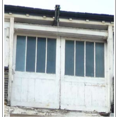
EXTERNAL VIEW OF WINCH
