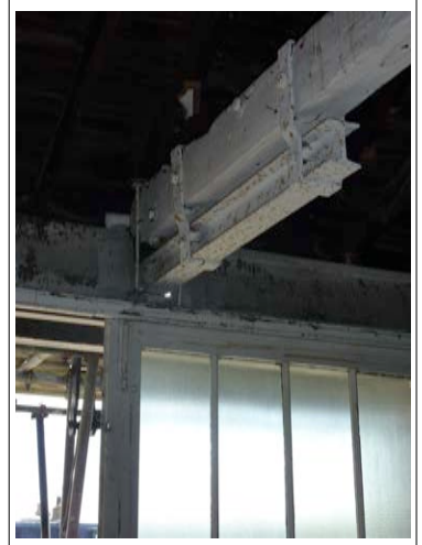
INTERNAL VIEW OF WINCH
