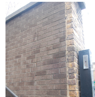
Inside view of retaining wall to 100 Chalk Farm Road showing how wall has been reduced in depth and rebuilt
