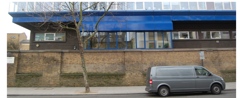
Section of same retaining wall from street showing it lowered and rebuilt
