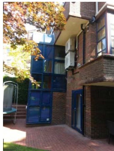
Air Conditioning units (West Elevation)
