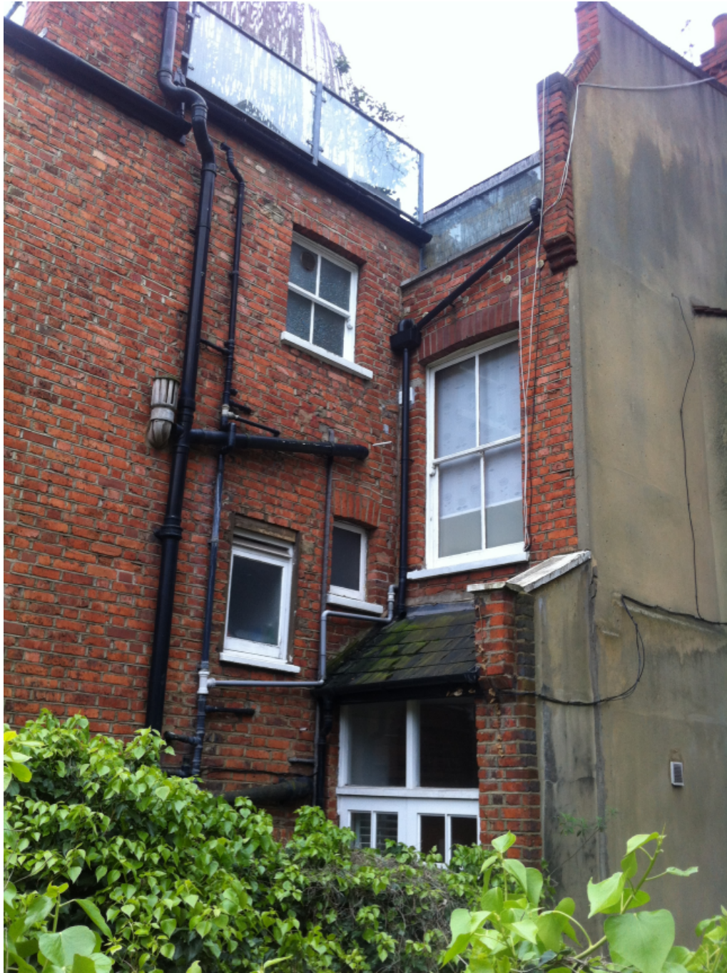
The rear of 31 Holmdale Road and the flank wall onto which the proposal would be constructed.
