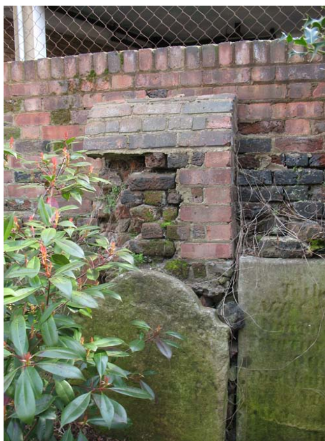
Photograph 4: Pier B not full height with missing bricks
