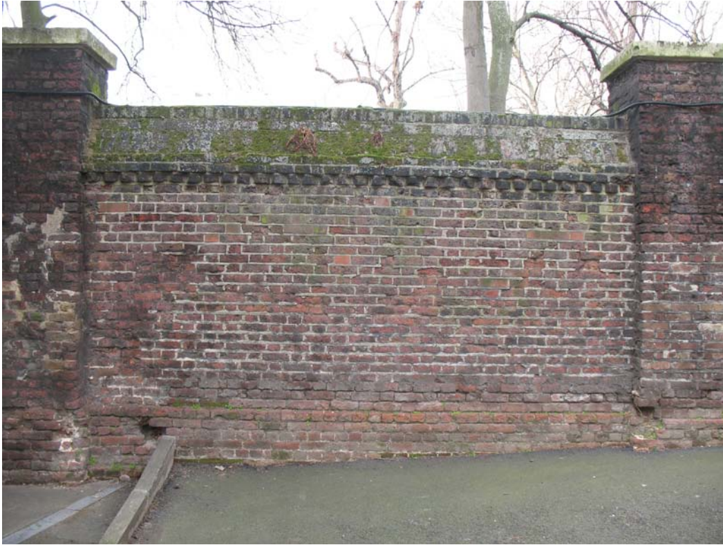
Photograph 23: Wall panel 28 showing missing bricks in panel and adjacent Piers
