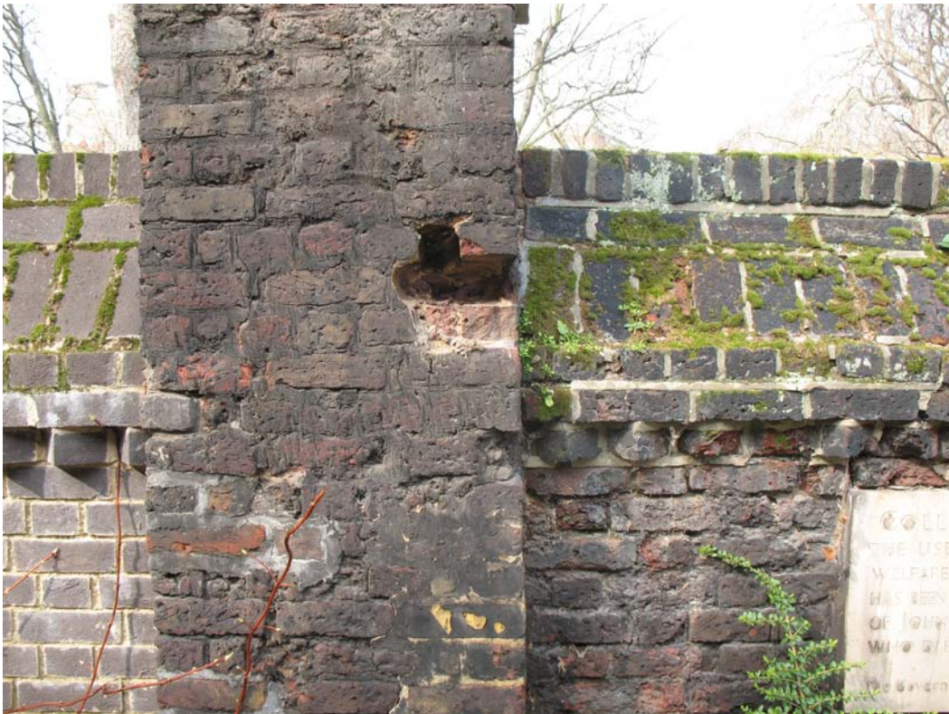
Photograph 20: Missing bricks to Pier X
