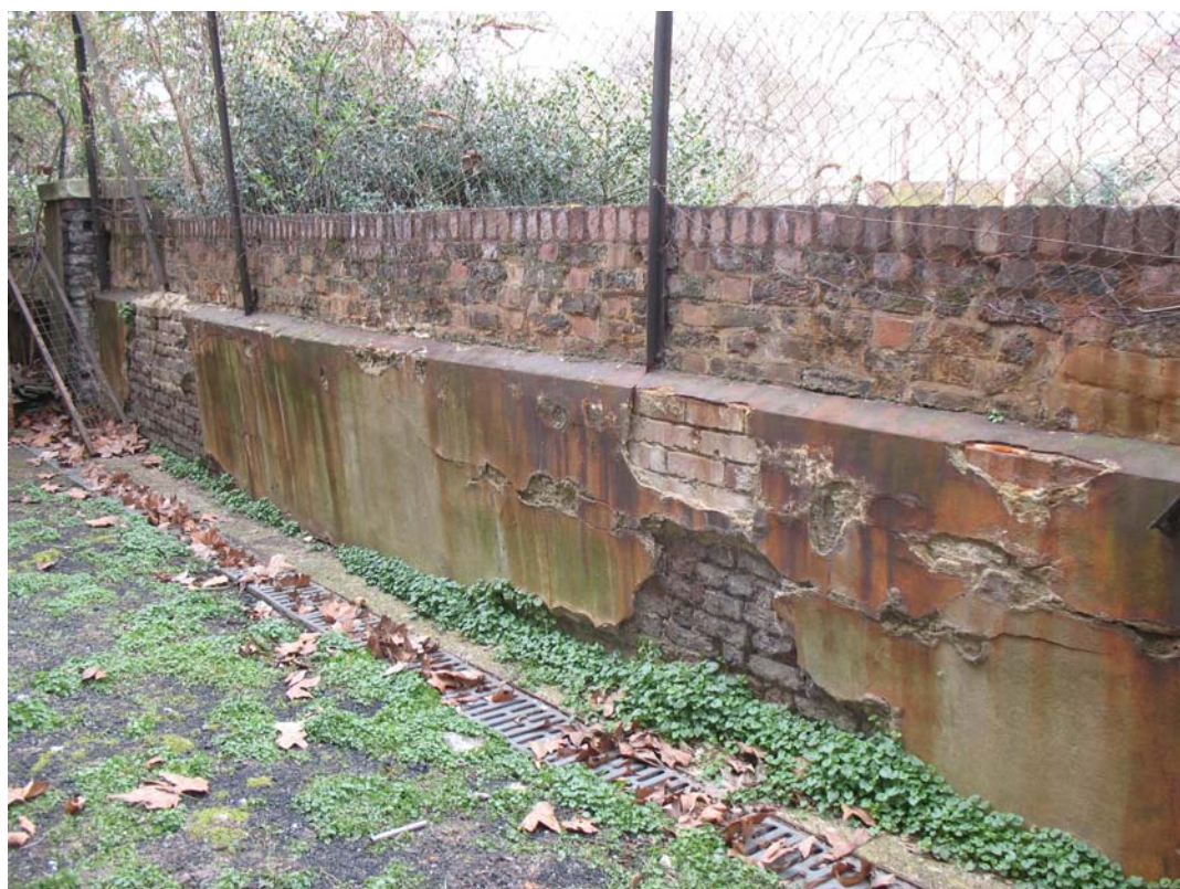
Photograph 12: South elevation of wall panel 1 & 2 showing failing render
