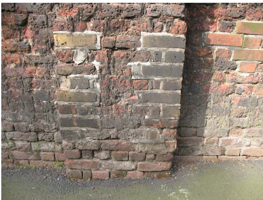
Photograph 22: Pier AA with poorly stitched in brick repairs
