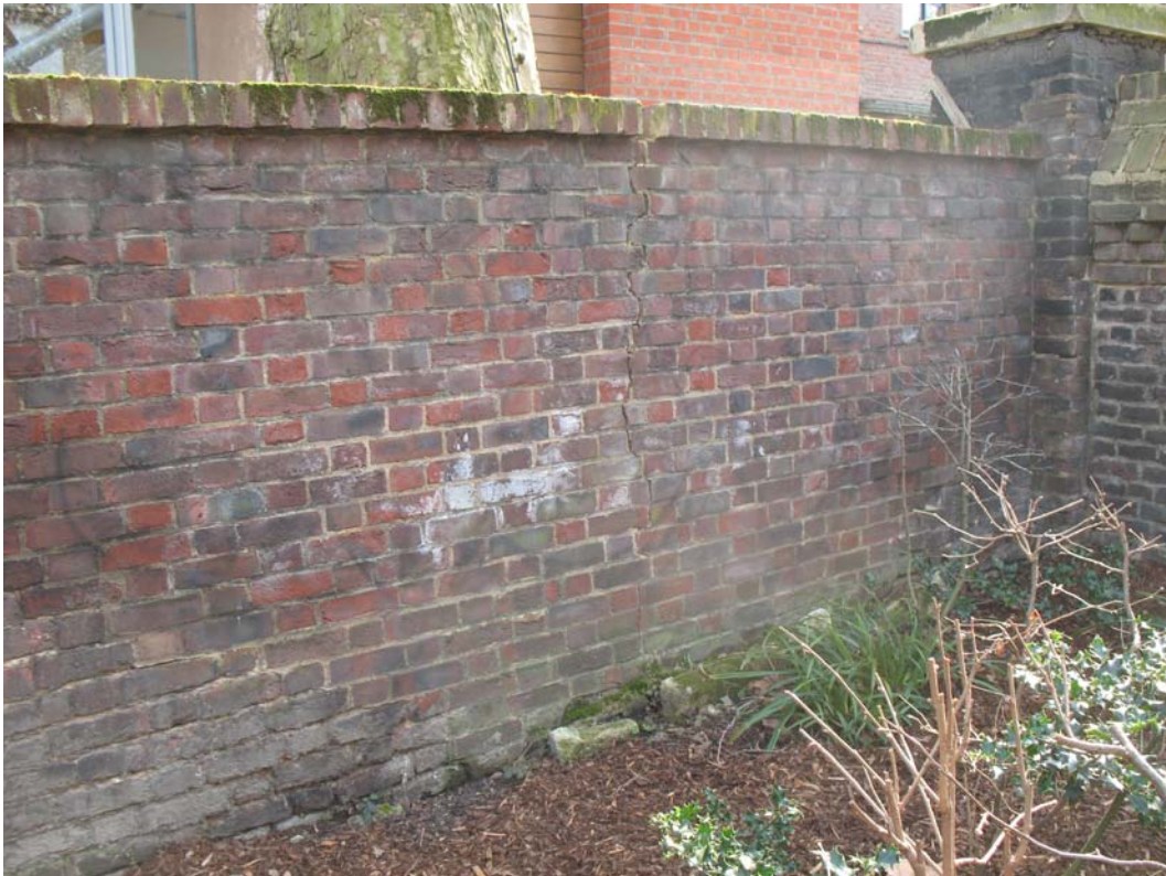
Photograph 8: Vertical crack in panel 18 in location of tree. Panel has been reconstructed
