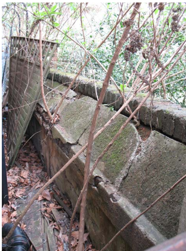
Photograph 14: Wall panel 3 showing failing render
