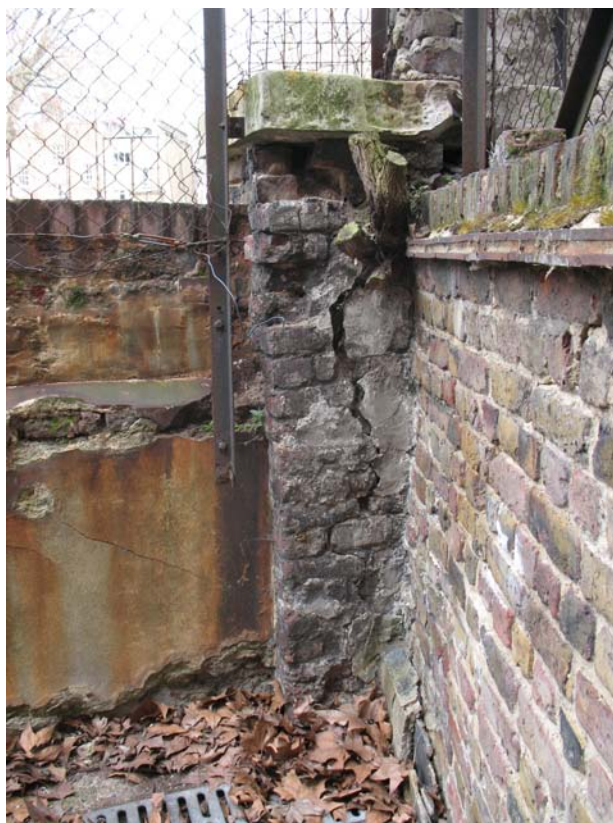
Photograph 13: Pier A showing cracking and cut back stump embedded in wall
