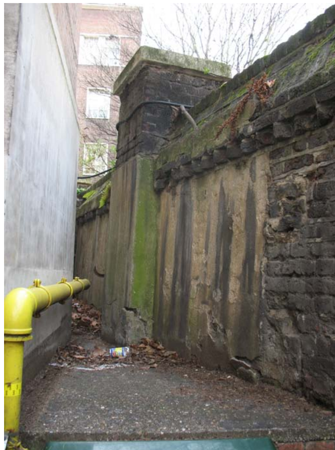
Photograph 24: Cracking render to Wall panels 29 and 30
