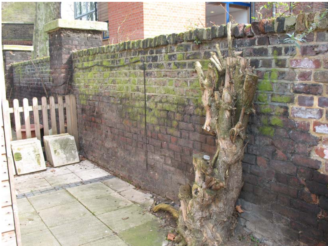
Photograph 10: Wall panel 20 with loose brick on edge course and close proximity of cut back tree.
