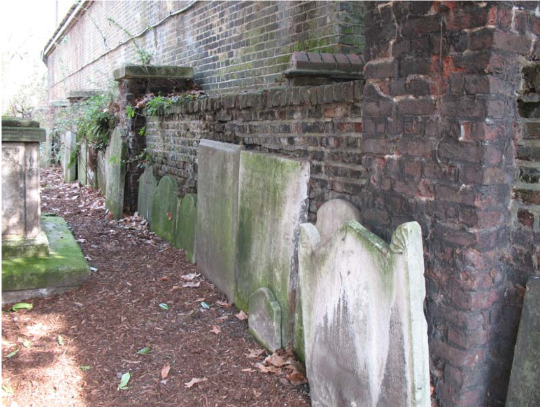
Photograph 7: Wall panel 14 leans toward garden in location of return wall on other side
