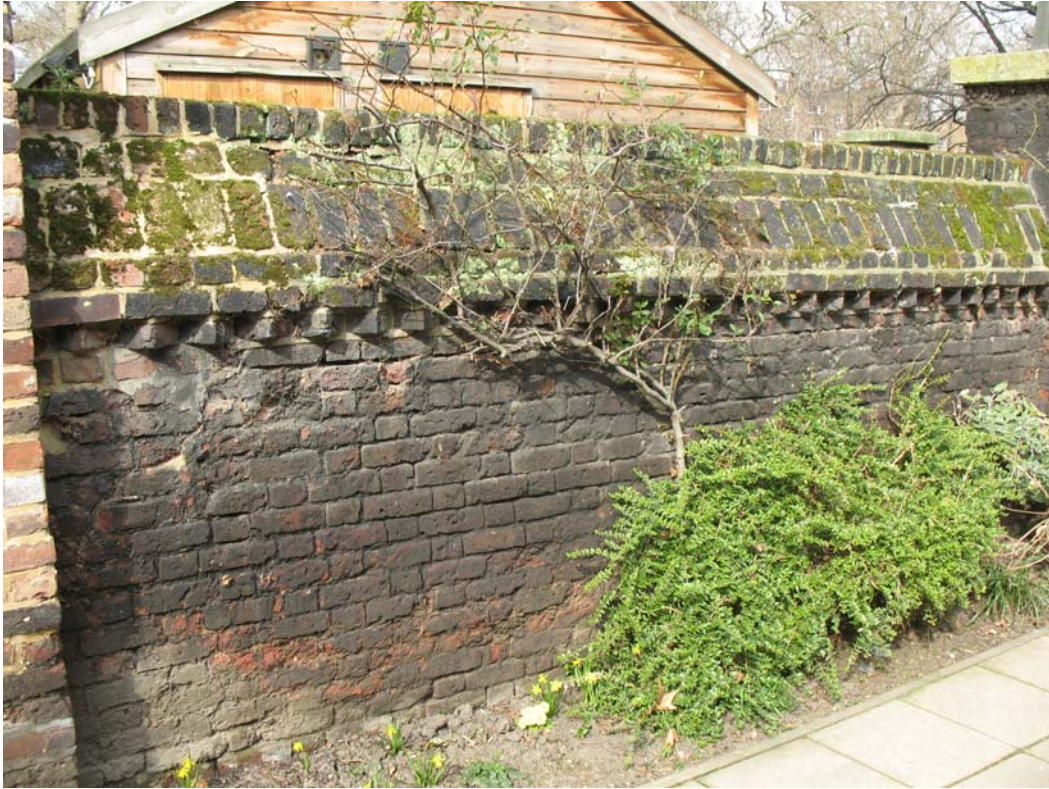
Photograph 19: Wall panel 20 with eroded dog tooth course and diagonal crack adjacent to Pier U
