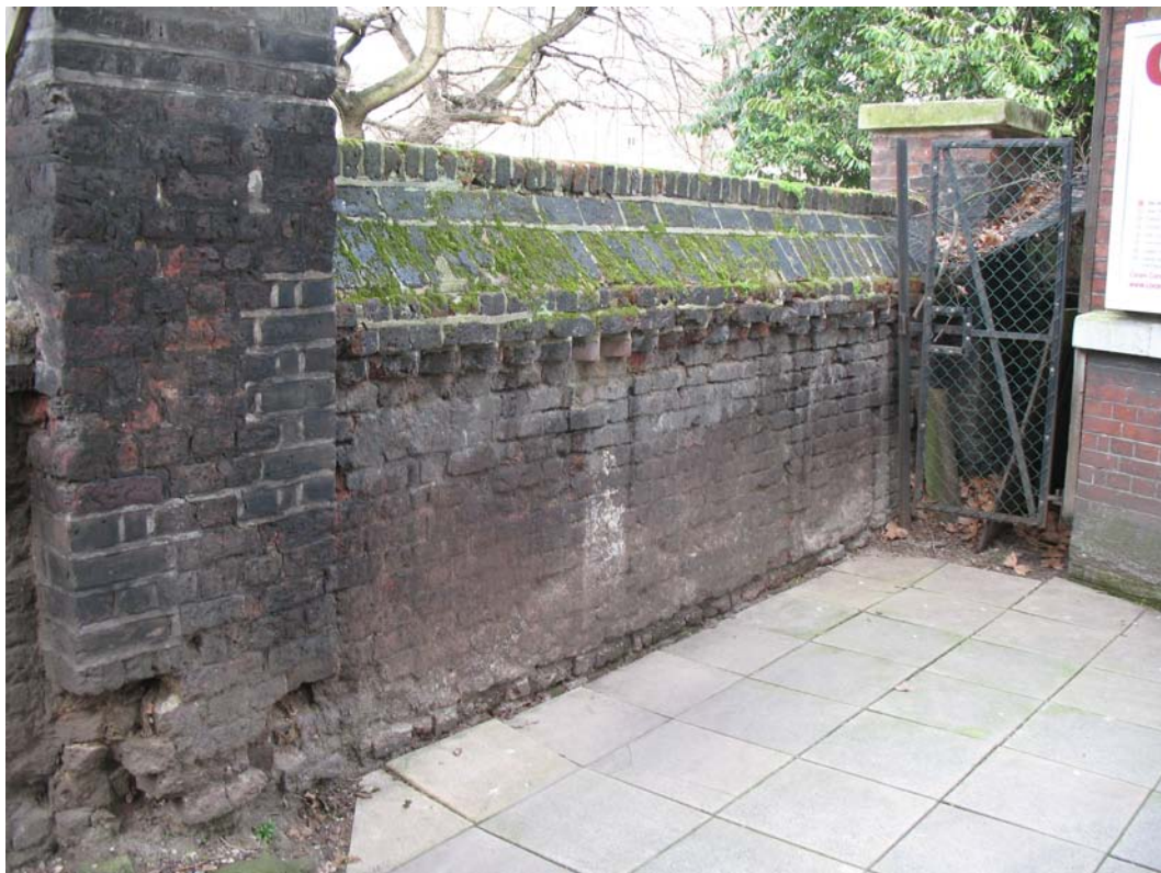
Photograph 16: Missing bricks to base of Pier R and general condition of Wall 17
