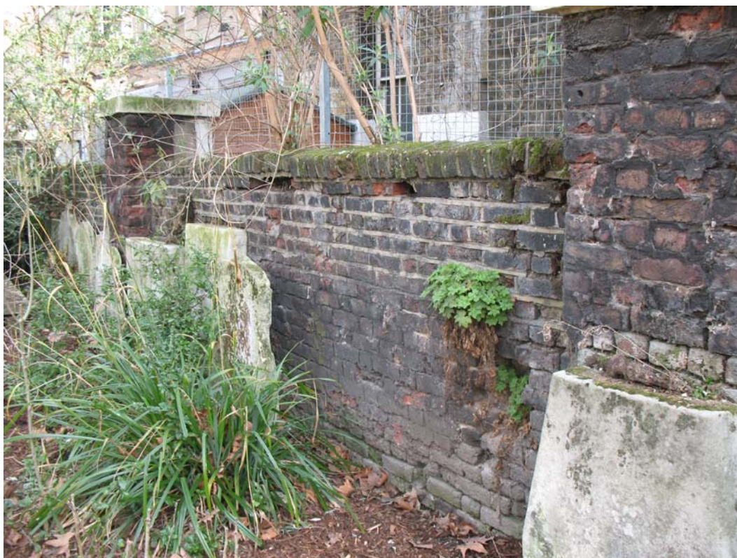
Photograph 5: Wall panel 9 with missing bricks and vegetation growing in holes
