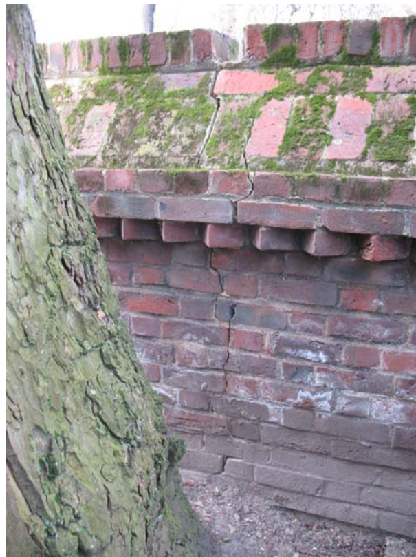
Photograph 18: Vertical crack in Wall 18 and missing coping brick on edge
