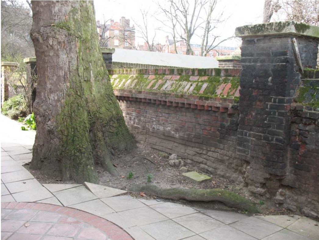
Photograph 17: Large tree in close proximity to Wall 18 which has a vertical crack. Missing bricks also in base of Pier R.
