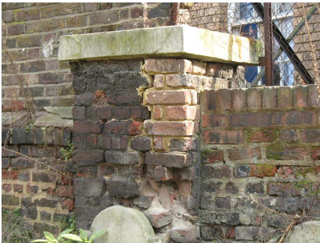
Photograph 3: Pier A showing poor quality local reconstruction and missing bricks
