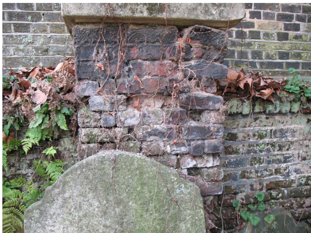
Photograph 6: Pier N in particularly poor condition
