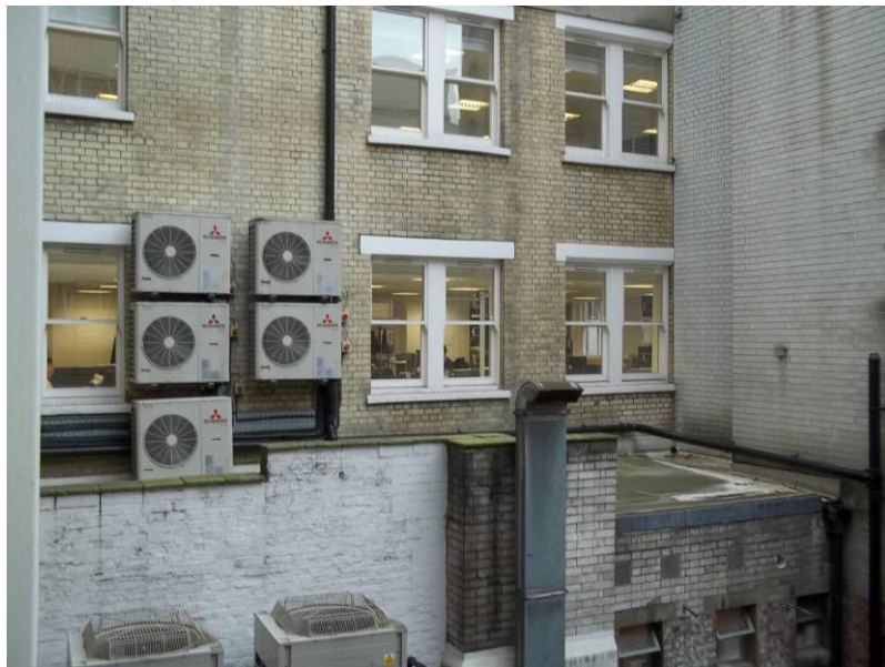
Photograph 2 - 29 - 30 High Holborn - Rear Elevation Existing Ventilation plant and flue
