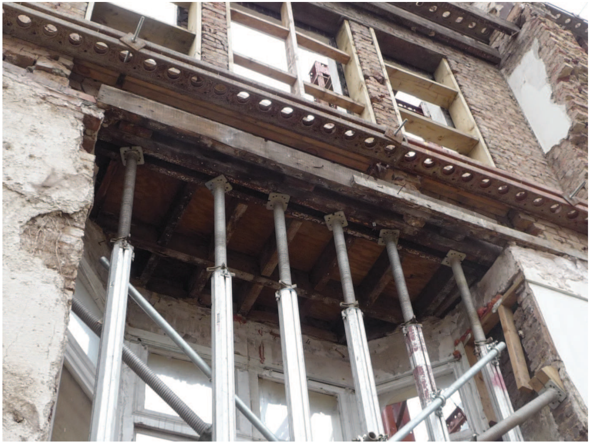
Photograph 12: Rear face of retained facade to No.44 showing RSJ's propped and timber bay window flat roof.
