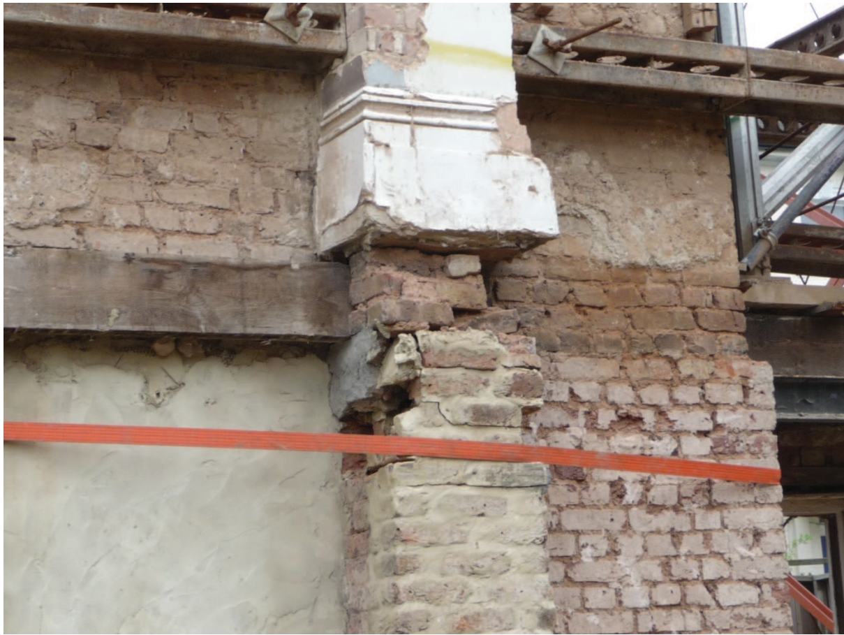
Photograph 14: Rear face of retained facade showing very poorly bonded masonry with embedded timbers and unstable pier remnant.
