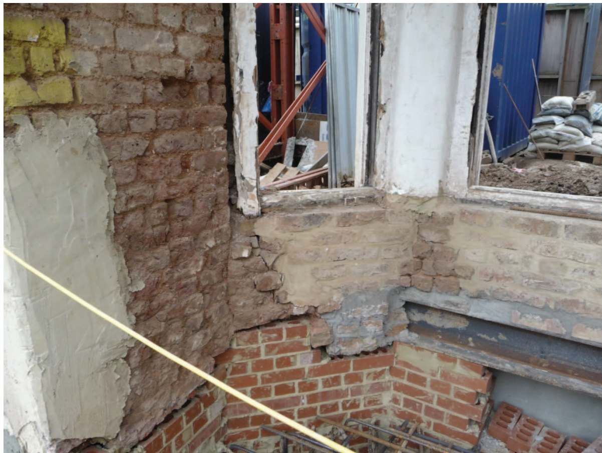
Photograph 15: Rear face of retained bay projection, showing poor quality masonry and minimal bonding.
