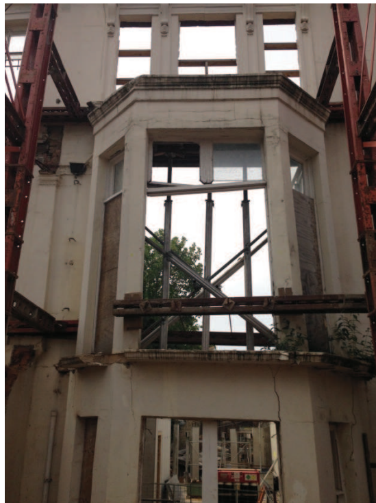
Photograph 19 Showing typical condition of No.45 bay windows, suffering distortion
