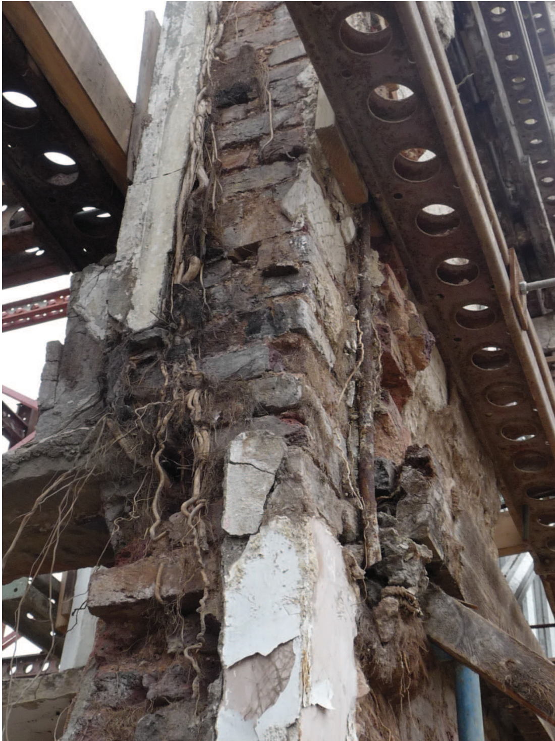
Photograph 16: End view of facade. Embedded roots and vegetation with very poor masonry
