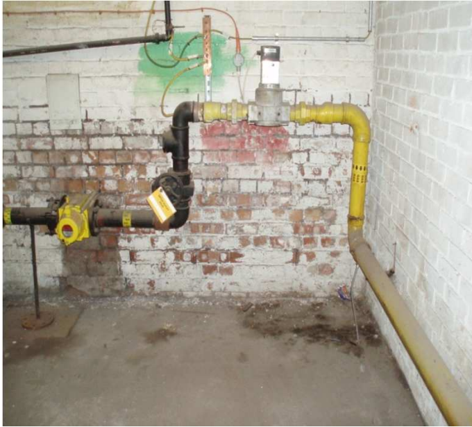
Image 9: Staining in Boiler Room
