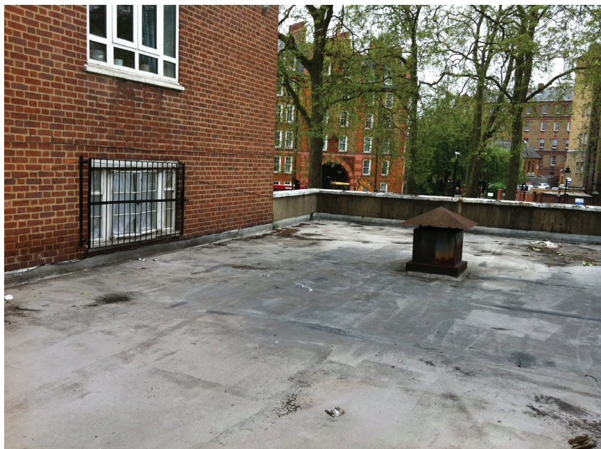
Obstructed View. Window to existing flat, to be blocked
