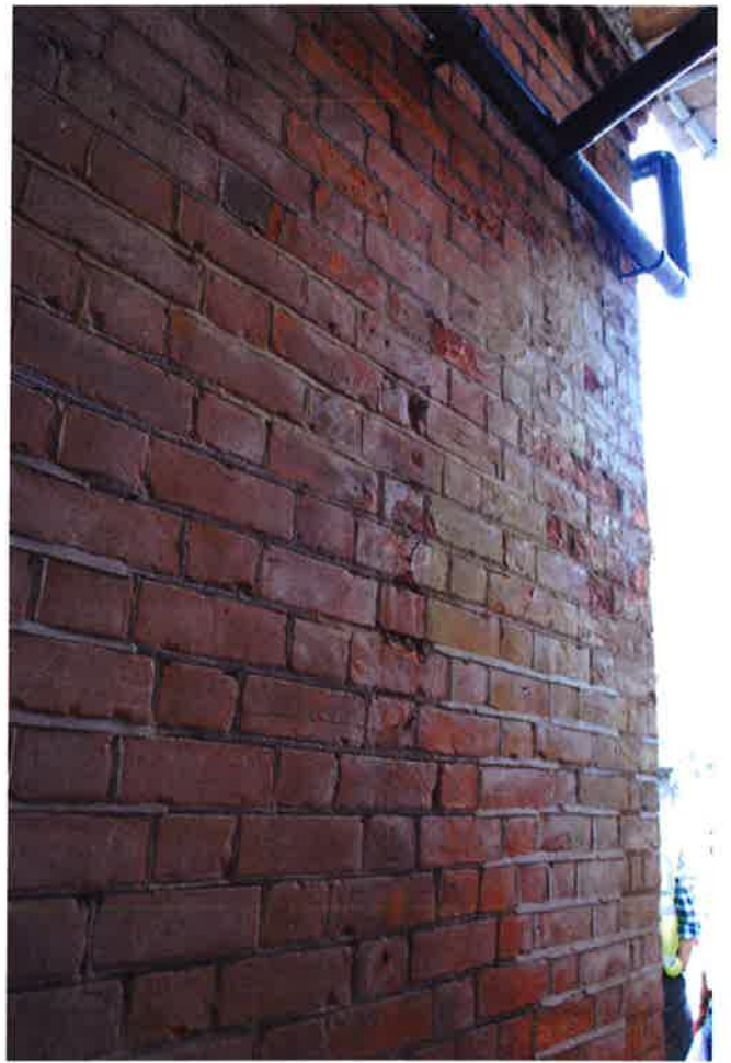
pointing problems and spalling10.JPG
