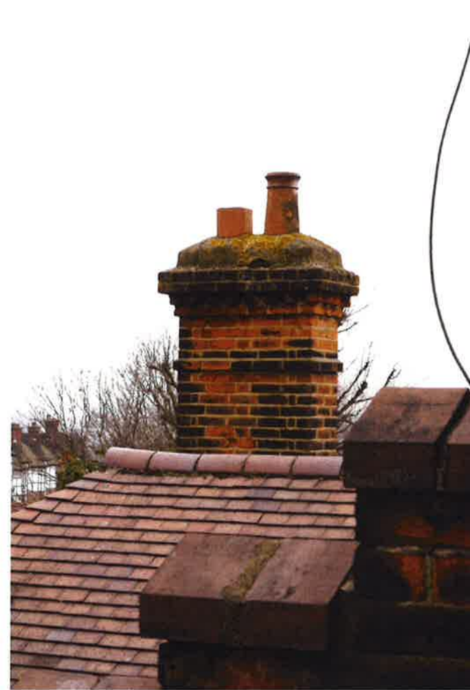
Existing Chimney Stack at 4 Clorane Gardens (replacement to no. 2 has been detailed to match this)
