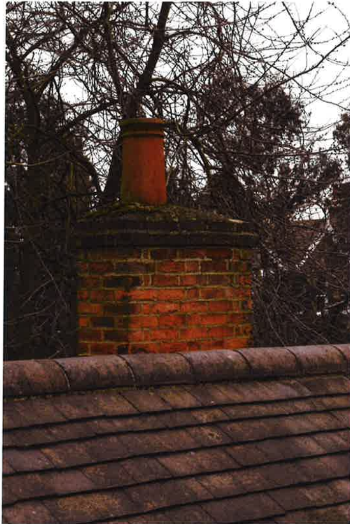
Existing Chimney Stack at 2 Clorane Gardens (to be demolished and rebuilt) It is presumed that this was cut short at some point in time and originally matched that at no. 4.
