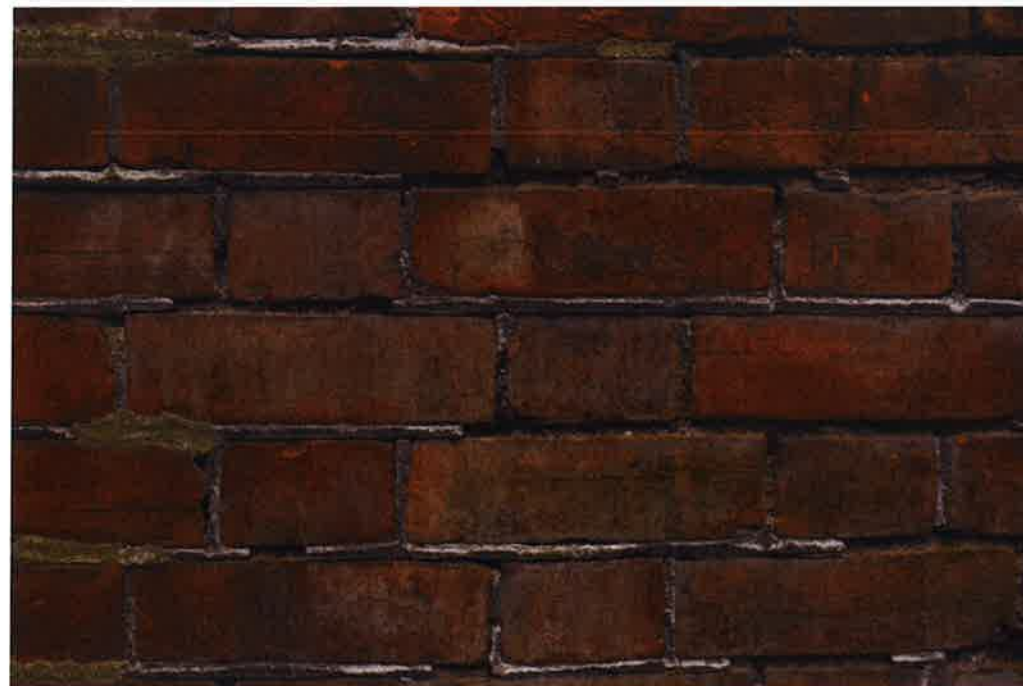
Existing Brickwork at 2 Clorane Gardens showing areas of original pointing which will be reproduced as best as can be achieved
