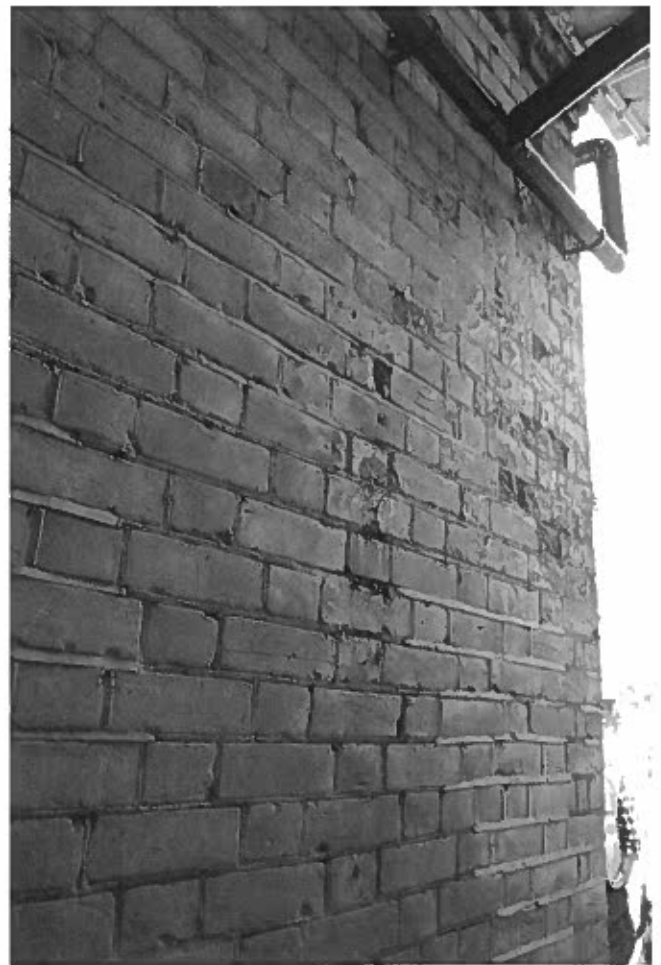
pointing problems and spalling10.JPG
