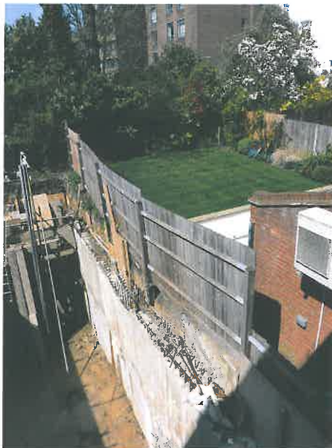
View of recent basement excavation to rear 8 Antrim Grove. Water in base of excavation is rainwater.
