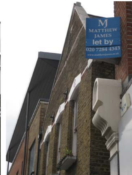
Bowing Gable Wall
