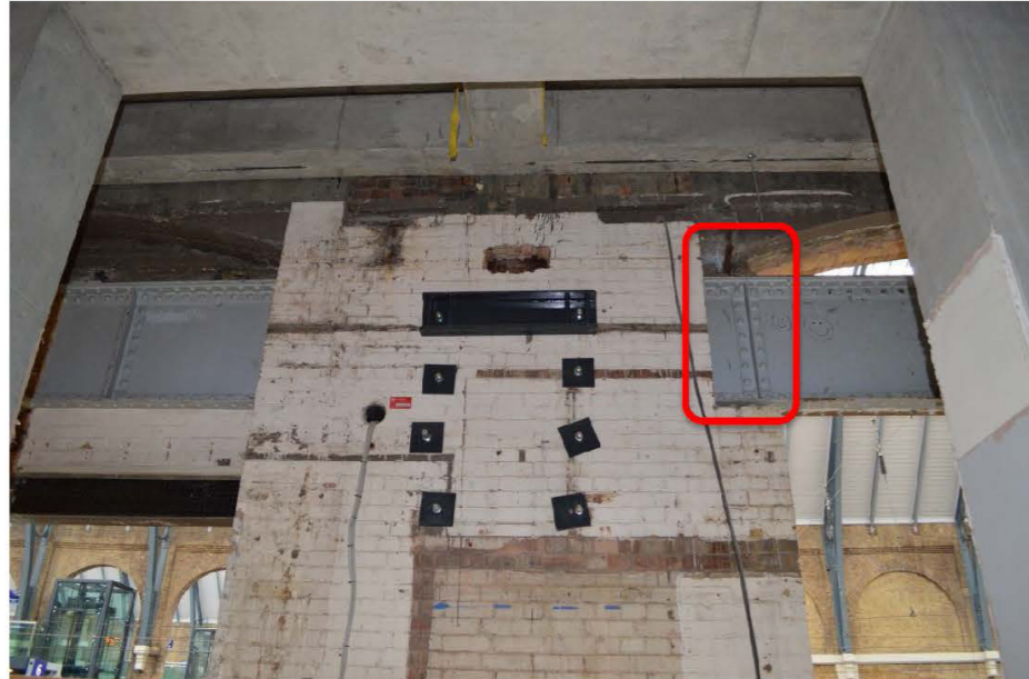
Figure 6: Rear view of connection between steelwork supporting clock and masonry pier. Image shows archway 1 on left hand side and archway 2 on right. Brickwork appears to have been removed around plate girder beam (in red).
