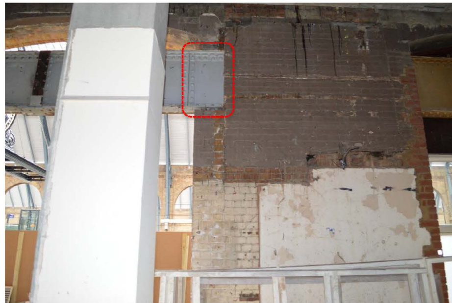
Figure 11: Masonry pier adjacent to central opening with brickwork removed around plate girder beam. Similar detail at other end.
