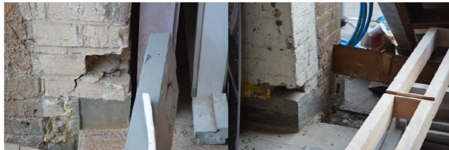
Figure 7: Individual brick removed near base of piers of central opening. From left image, crack noted emanating from removed brick.
