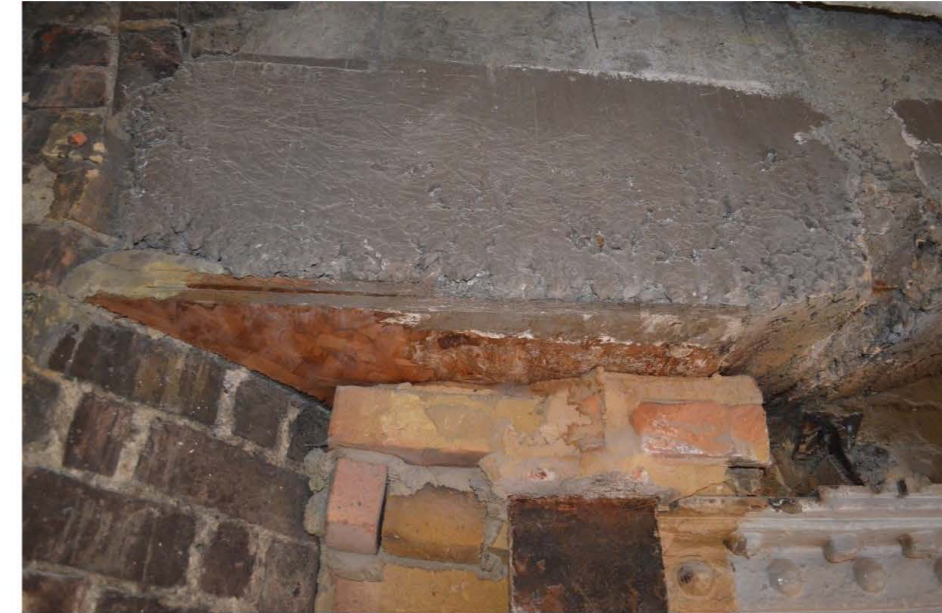
Figure 4: Close up of connection detail at left hand end of concrete arch
